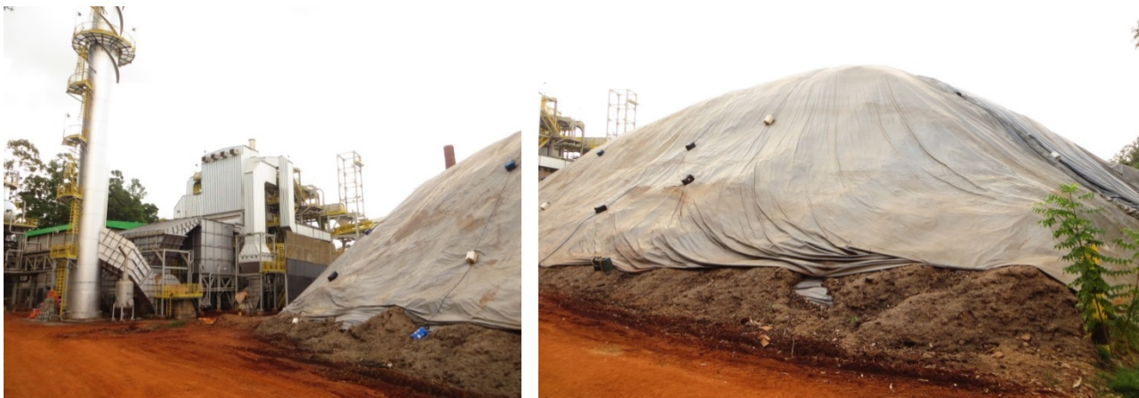
Figure 20 - Left: steam boiler for firing bagasse, Right: stored leftover bagasse from previous season. Araras, São Paulo
